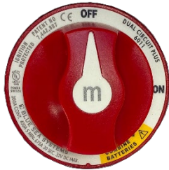
Battery Isolator Switch 'Off'
