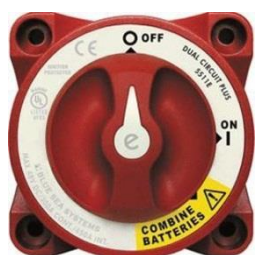
Battery Isolator Switch 'Off'
